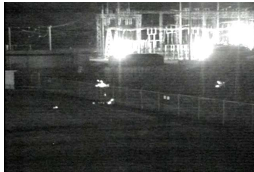
Surveillance video screenshot Metcalf Substation April 16, 2013
